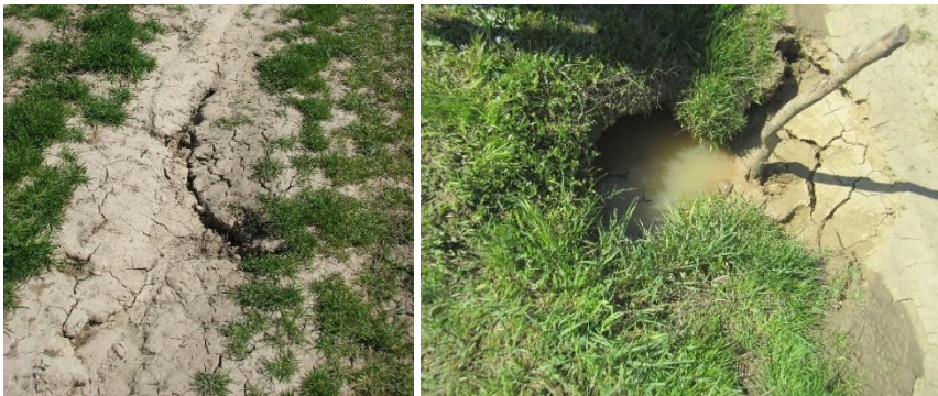
Figure 3. Surface cracking of a dike, and erosion hole on the edge of the dike crest
